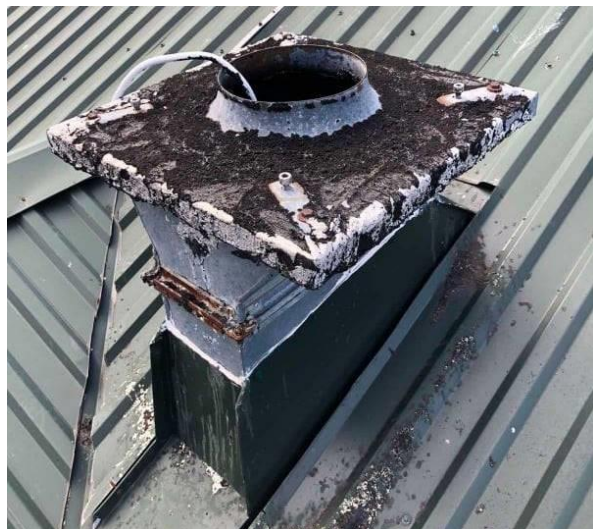
Nedostatak ventilacione kape/ Lack of ventilation cap trim
